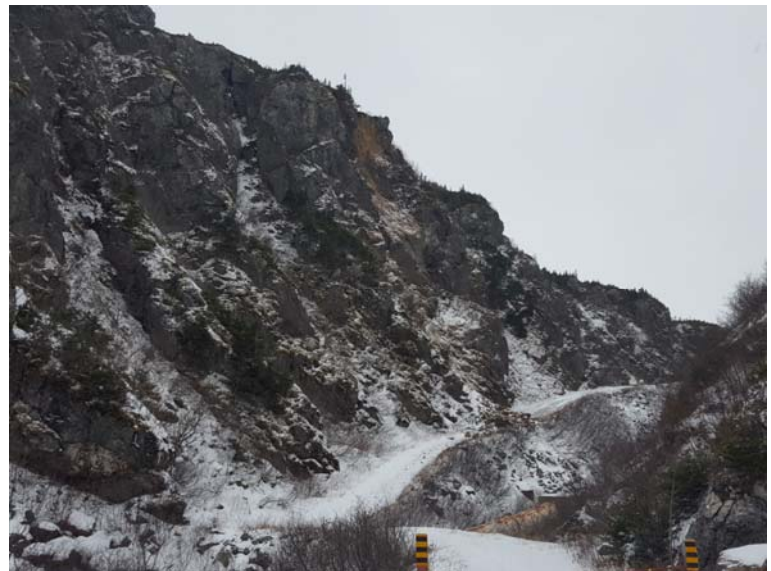
Photo 6 – Scarp on rock slope of fall area.
