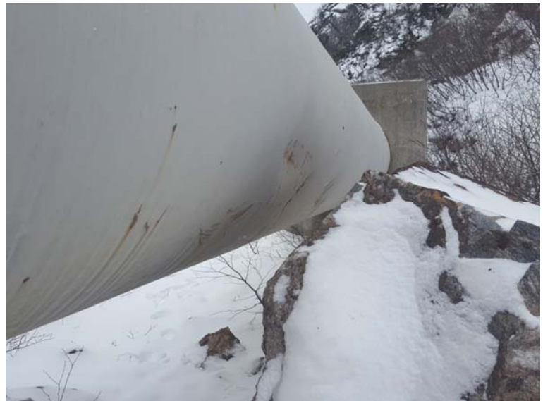
Photo 16 – Impact Area 3. Approximate 5 tonne boulder impact.
