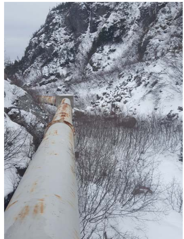
Photo 10 – Debris Field below the access road.
