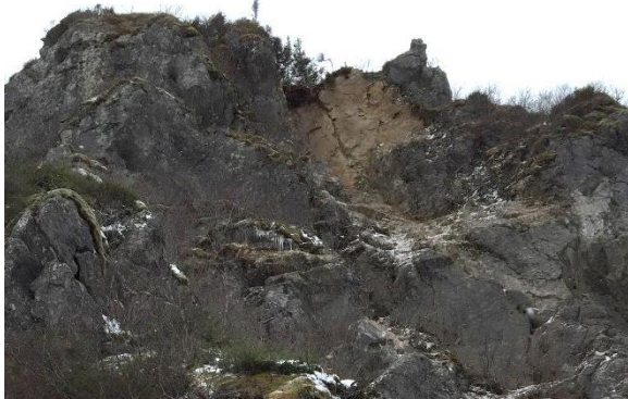
Figure 6 – Unstable Rock Slope
