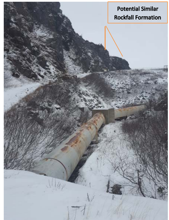
Photo 2 – Rockfall area from the culvert crossing.
