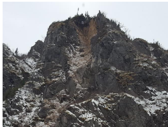
Figure 7 – Unstable Rock Slope
