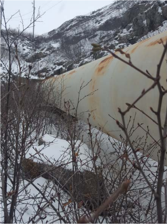
Photo 13 – Impact Area 1, approximate 2 tonne rock at base of penstock.
