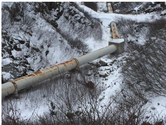
Figure 4 – Overview of Damaged Area
