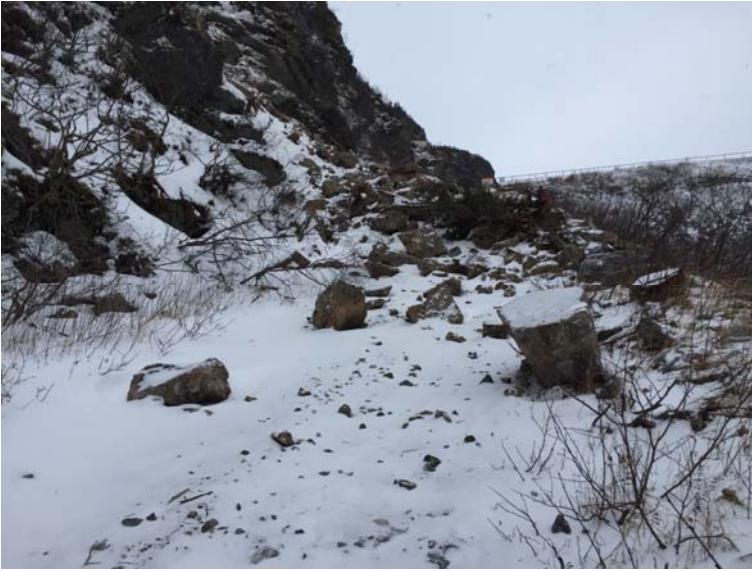
Photo 5 – Debris field on access road looking towards dam.
