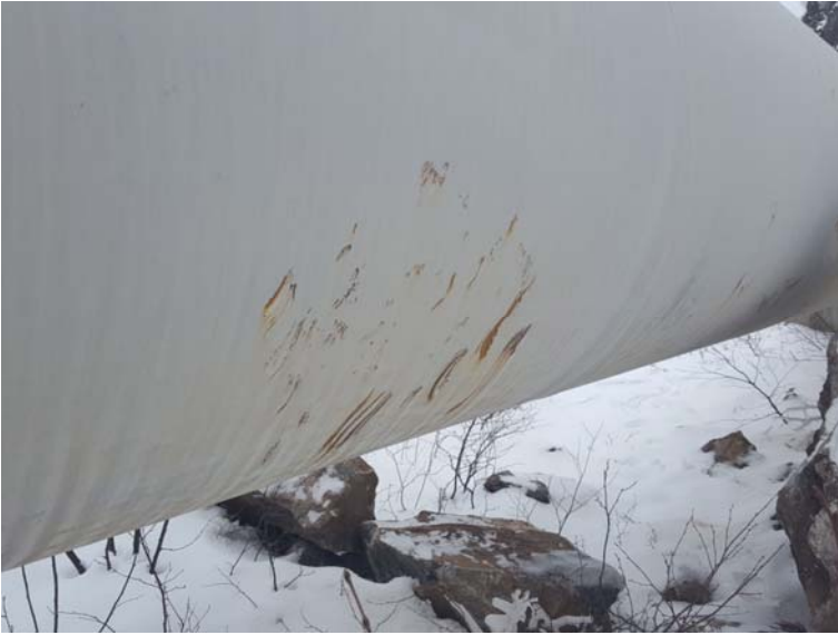
Photo 15 – Impact Area 2, paint damage, steel indented.
